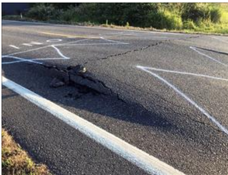
Buckling road from excessive heat, State Route 544 near Everson, Whatcom County, June 28, 2021
