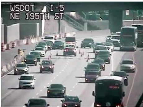
Buckled northbound Interstate 5 from excessive heat, near NE 195th Street, Shoreline, June 28, 2021
